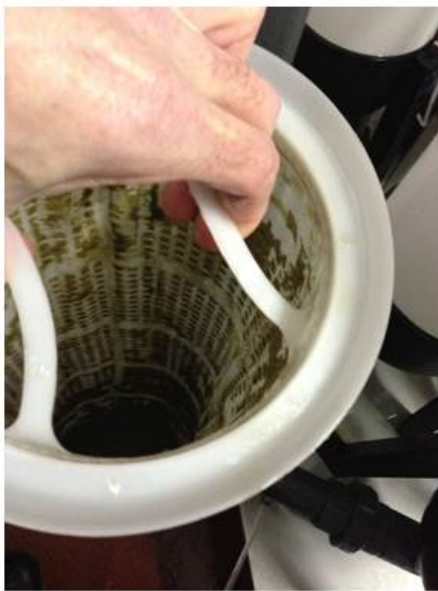
Mesh filter at the end of filtration run
