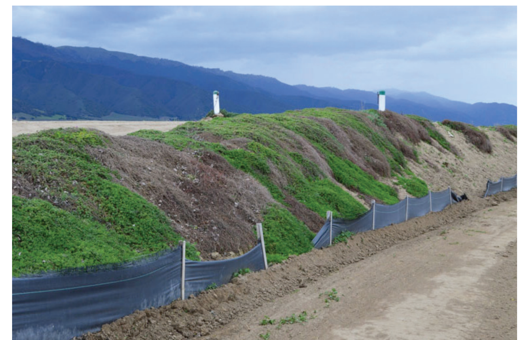
Figure 2. Traditional silt fence exhibiting wind damage, originally installed to exclude frogs and other wildlife from the growing environment.
